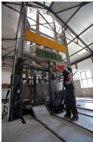
Figure 80. The oldest functioning elevator in Slovenia in the Coal Mining Museum of Slovenia [Photo: Premogovnik Velenje].
